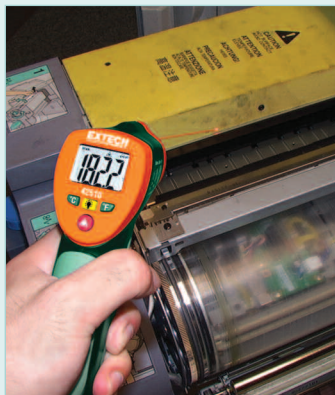
Electrical Troubleshooting for hot spot detection
